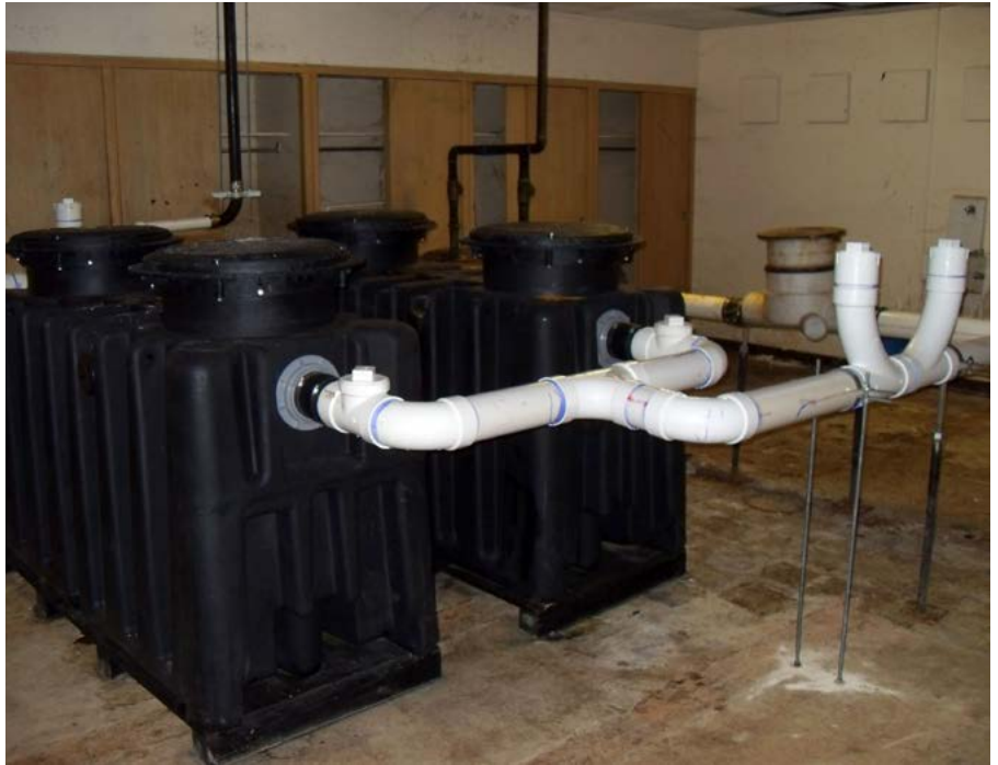
Two Endura® XL100 Grease Interceptors, (which could fit in the back of a pick-up truck), were installed in parallel configuration.
