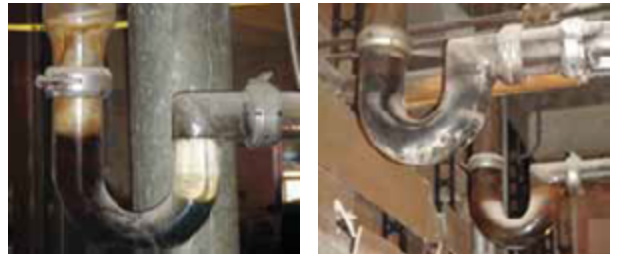
Crud buildup from years of operation are clearly visible in glass waste lines
