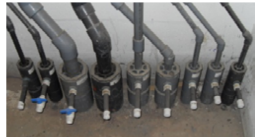
The IPEX Guardian™ Vinyl double-containment system was required for underground runs, which transitioned to IPEX single wall PVC and Corzan CPVC inside the facility.
