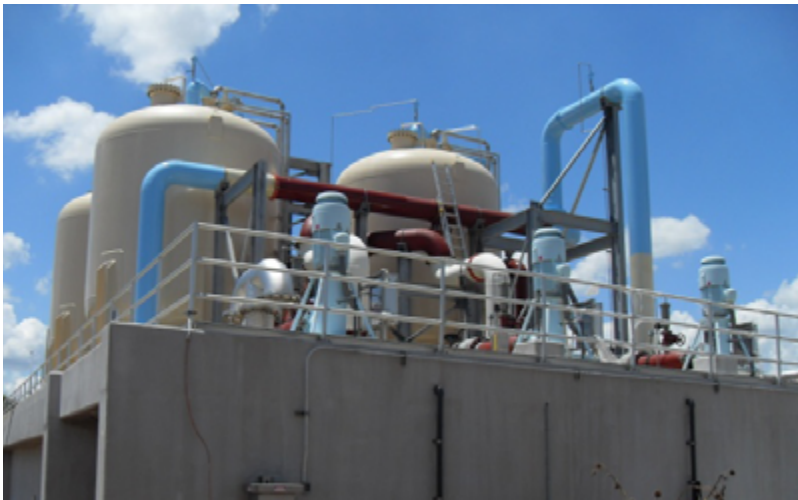
The City of Sugar Land Surface Water Treatment Plant delivers 9 MGD of potable water to residents.
