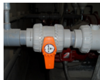
IPEX manual VXE, VX and electric actuated VKD Series Ball Valves were used throughout the facility to control flow as needed.
